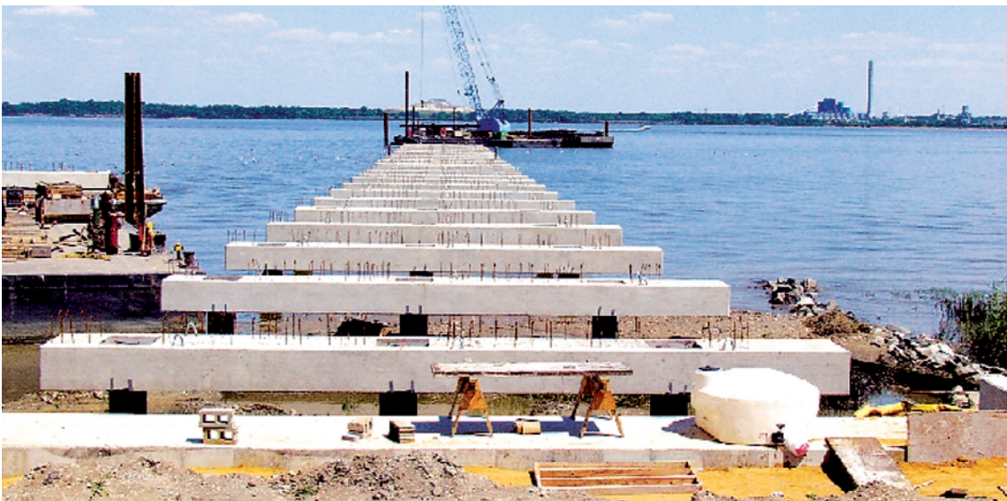
The construction of the Port of Wilmington’s dedicated automobile berth on the Delaware River is progressing on schedule with the placement of the support piles for the berth and pier caps. The berth on the Delaware River will be approximately 875 feet long, 115 feet wide and supported on 500 steel support piles.
